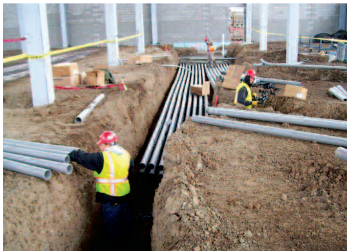
Four hundred electricians worked long hours to construct the 955,000-square-foot Chobani yogurt plant in Twins Falls, Idaho, in just 10 months.
